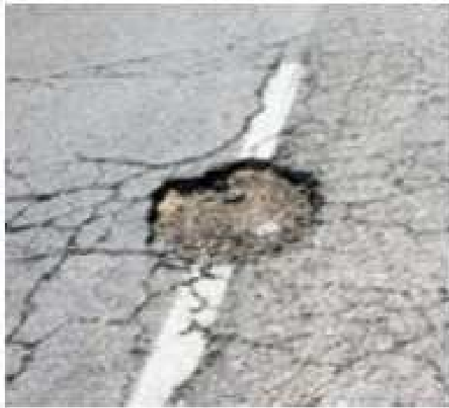
Figure 10: Typical small pothole with missing pavement.
